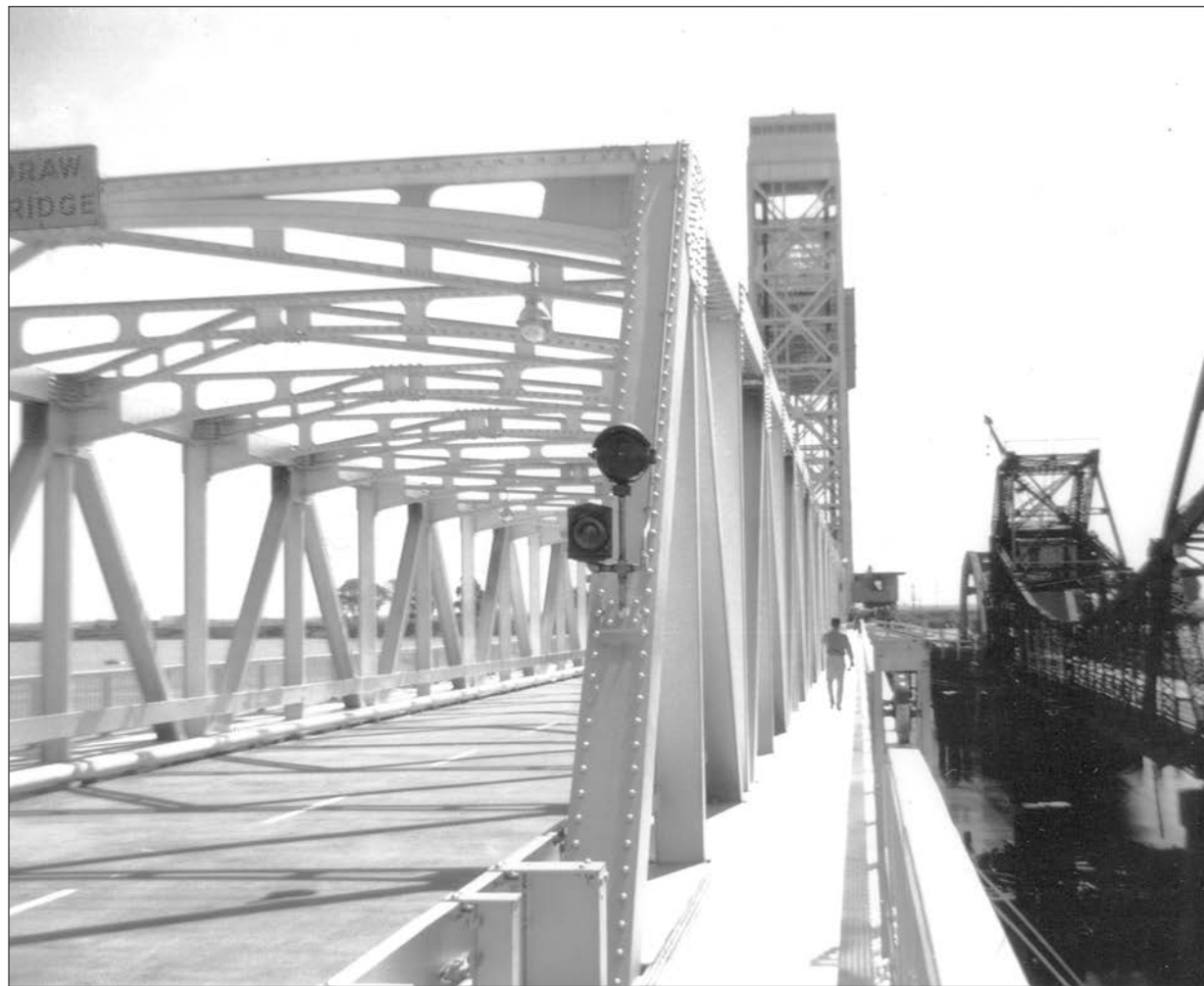
Rare photo of an old and new Rio Vista Bridge, late 1950's.
